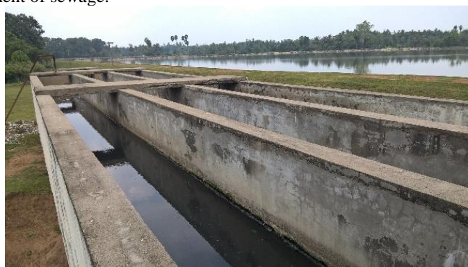
FIG (4) – TREATMENT UNIT
